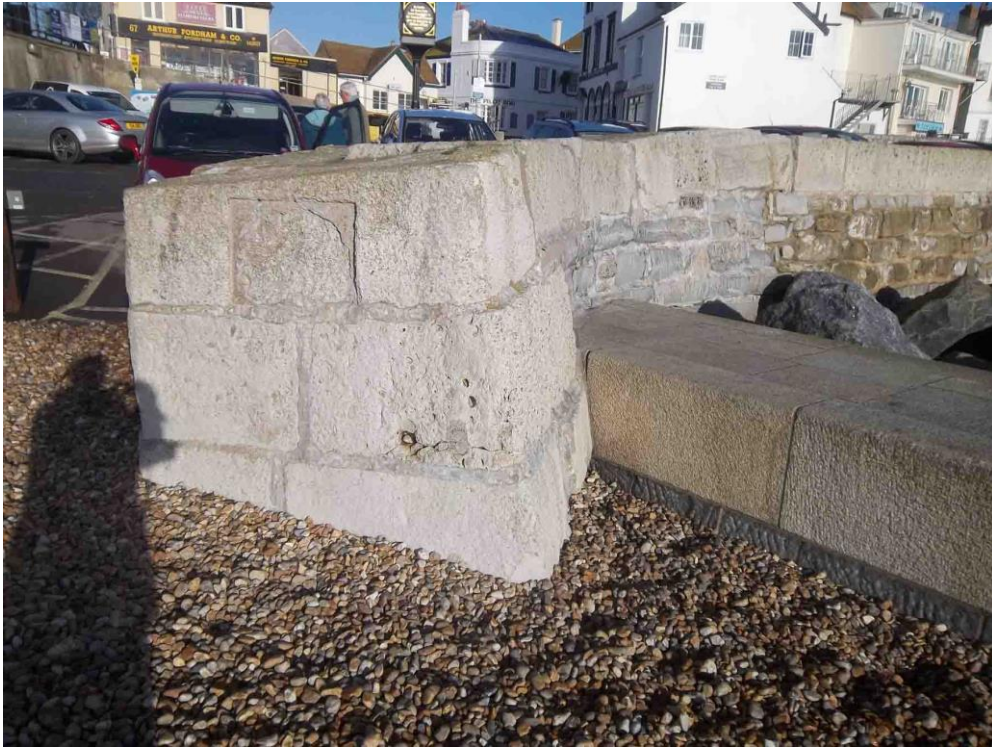
The termination of Cobb Gate Wall in 2014 – compare with the watercolour above. The old ramp to the beach lies under the tarmac and shingle. The old jetty continued from this termination, but the new jetty lies to the right. Cobb Gate Wall consists of Lias blocks under Portland Roach copings, but excavation of the beach to the right in 2005-7 revealed a host of repairs and old work of massive Portland blocks. The Lias work behind the start of the new jetty was put in after a major breach in the 1950s.
