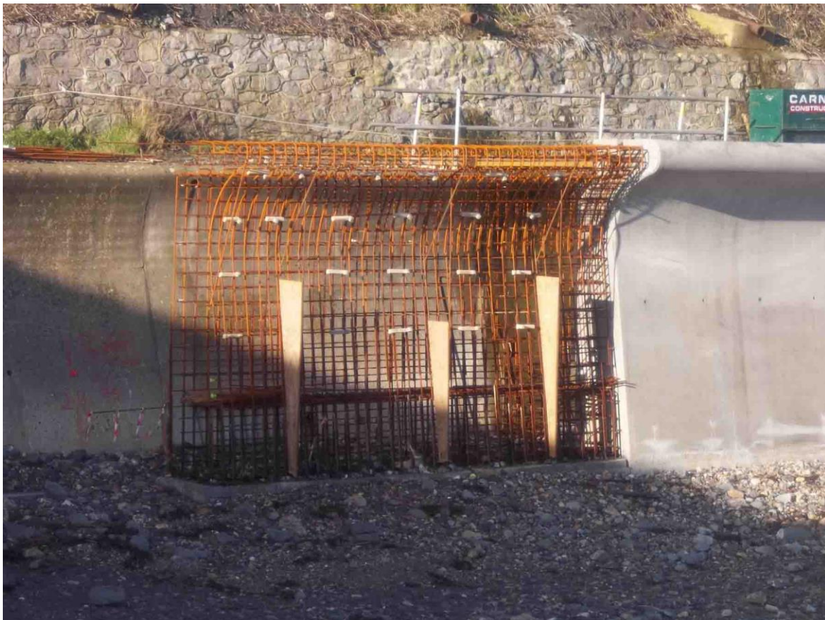
The new Church Cliff Wall under construction in December 2013, encasing the old
