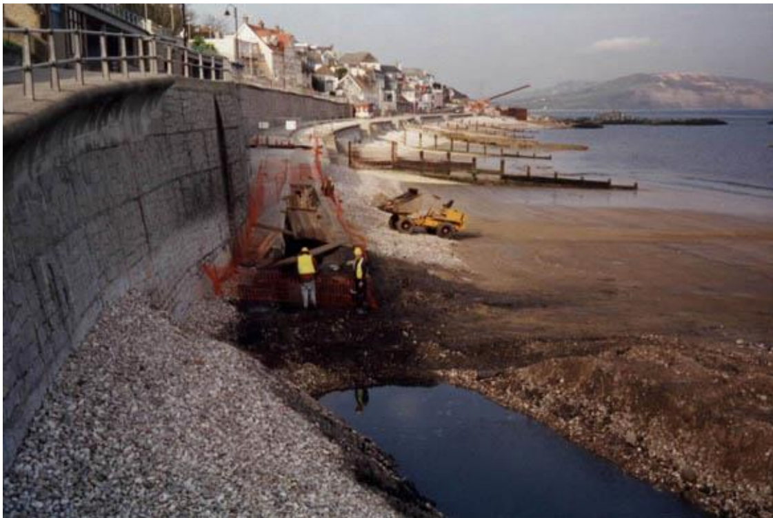
Marine Parade and the Cart Road Ramp in late 2005/early 2006 looking east. The 1978-9 walls supporting Marine Parade, the Cart Road and its ramp are in evidence. Foundations are being dug for a new Cart Road Wall in the foreground to join up with that beyond the barricade. The beach level is low, despite some replenishment and groynes, but soon a new beach will be delivered. Close study reveals De La Beche's Jetty. In the distance a Norwegian barge stands off Cobb Gate Jetty with Larvikite boulders for the armour stone rockery at Cobb Gate. The central shelters are in place, shortly to be re-vamped.
