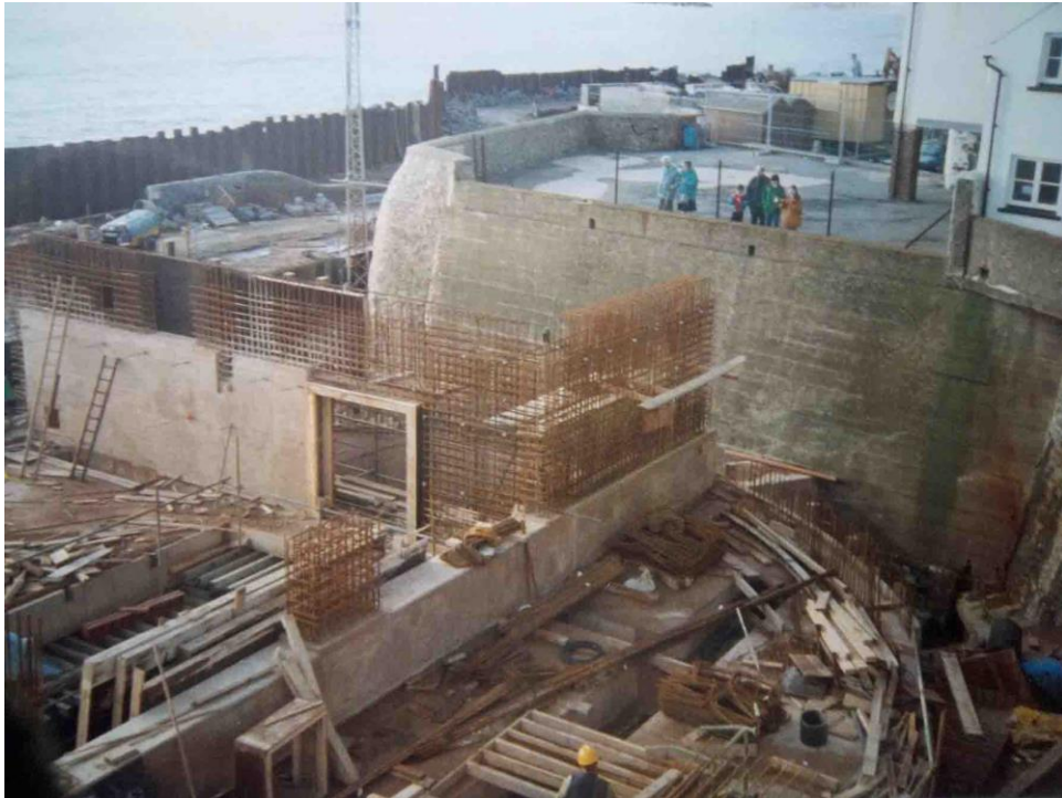
Gun Cliff cleared of housing, seen in 1993, with the Gun Cliff Sewage Pumping Station under construction on the beach in front. A coffer dam holds back the sea. Gaiche's Wall once sprung from the corner of Gun Cliff.
